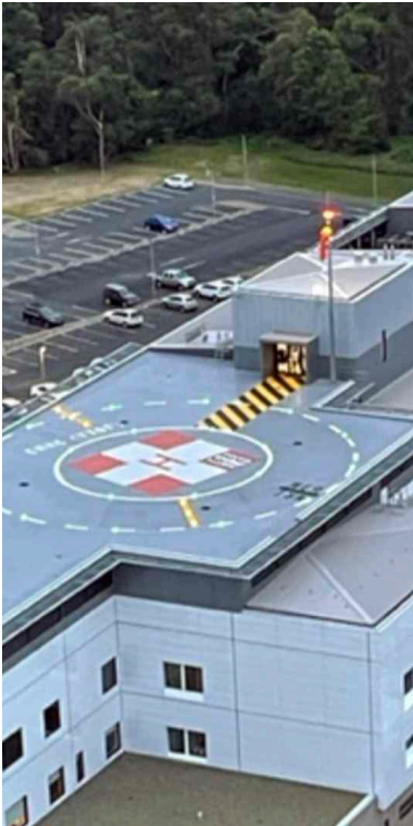
NSW Health - retro fit HLS IWDI Windsock assembly - North Coast, NSW
