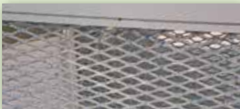
▼ Deteriorated polyester coating in 1996 after 6 years.
