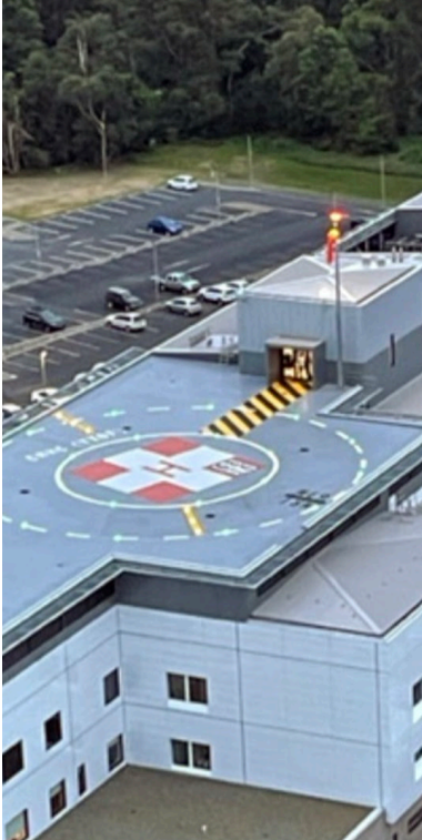
NSW Health - retro fit HLS IWDI Windssock assembly - North Coast, NSW
